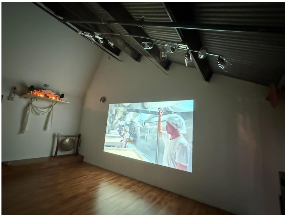
Audio and visual system in mezzanine
