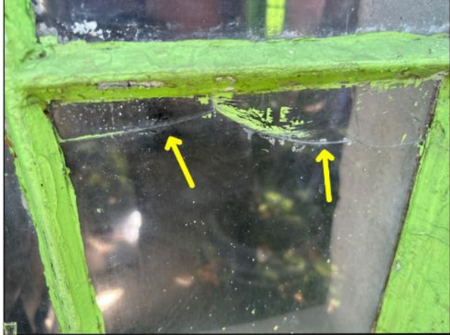
Cracked glass - needs to be serviced. At detached garage.
