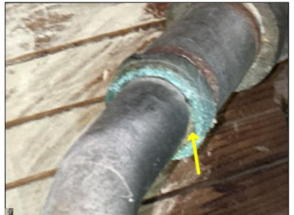
Corrosion is present at plumbing areas - this is a sign of slow leaking and should be further evaluated by a plumber. Half bathroom.
