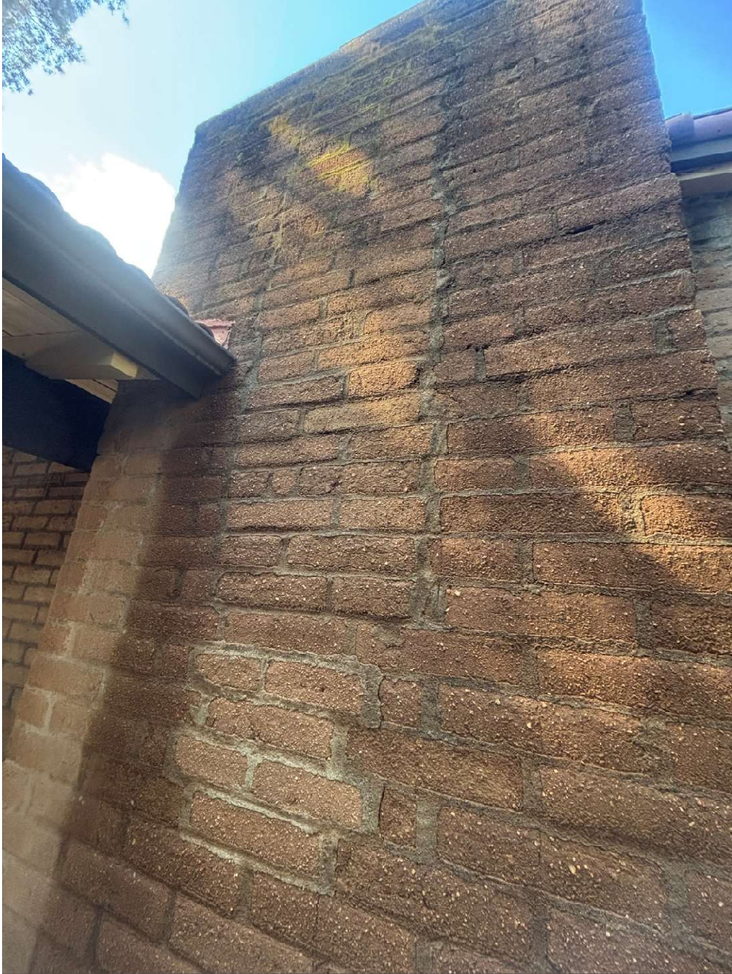
Previous Repair Work on Fireplace Exterior
